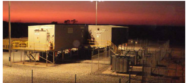
Lady Loretta Mine Power Station: Design, installation, testing and commissioning of 6MW standby power station and seven portable power kiosks.
