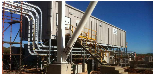
George Fisher Mine: 440V Crusher Switch Room
